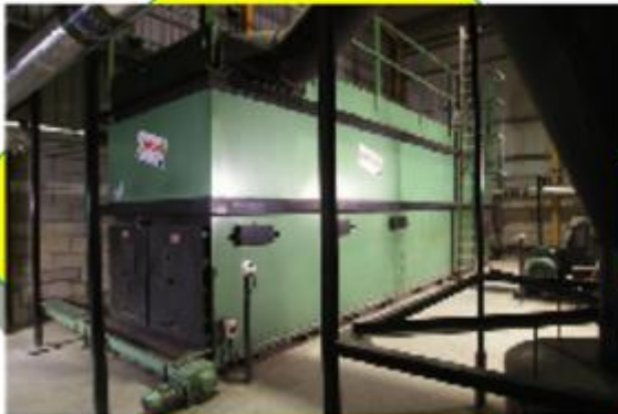
The Talbott C9 2,500kW Hot Water Unit
